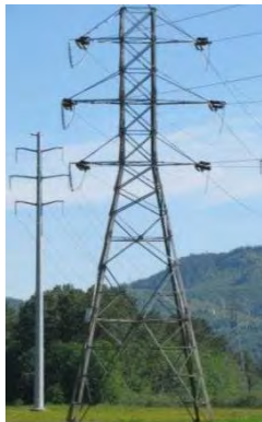
Transmission and Distribution
